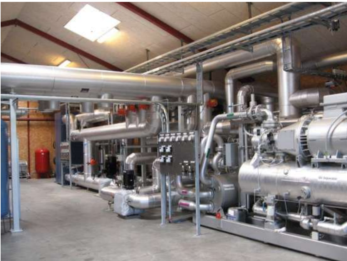
Fig. 6.16: Piping at the secondary side
