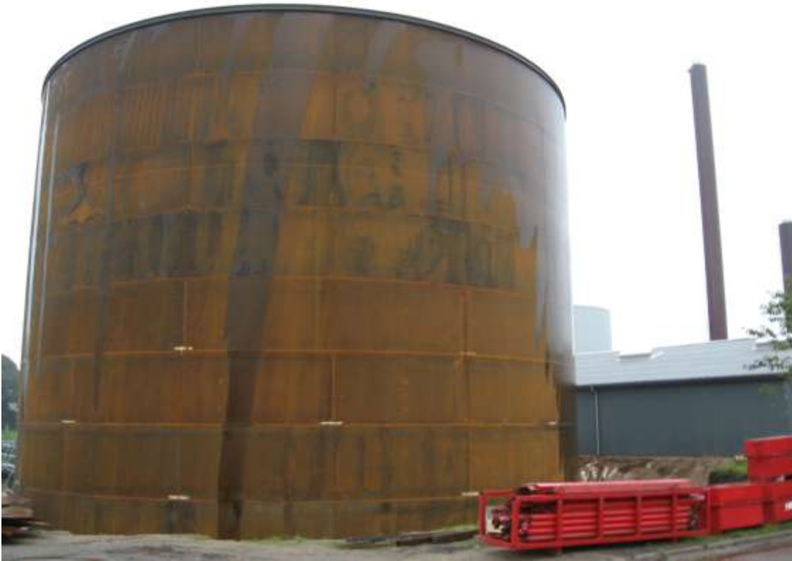
Fig. 6.10: Accumulation tank before insulation
