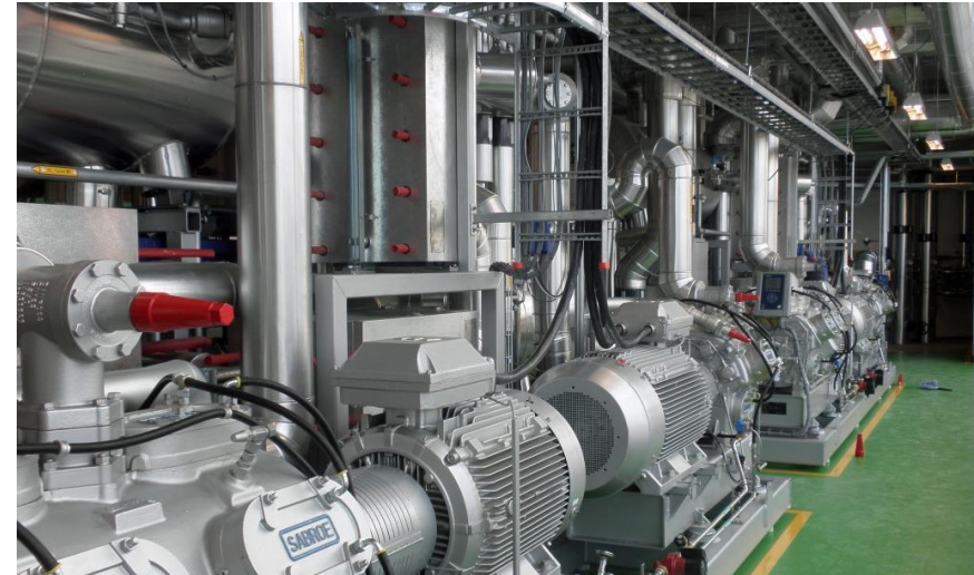
Figur 3.3 – Varmepumperne i Energicentralen i Bjerringbro.
