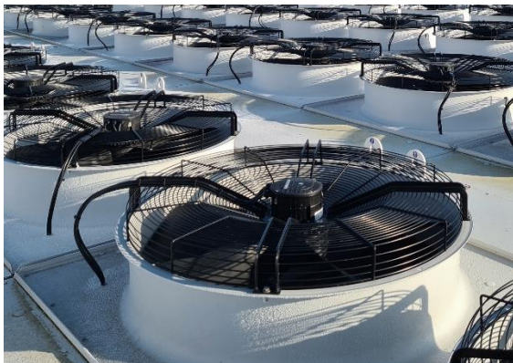
Figure 10. Close-up of the protective safety-grill on top of the fans of a flatbed evaporator.
